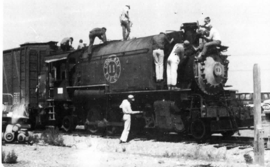
Like ants on a candy bar, Museum members clamber over 2-8-2T No. 11 to begin restoration work. (Dick Pennick)
